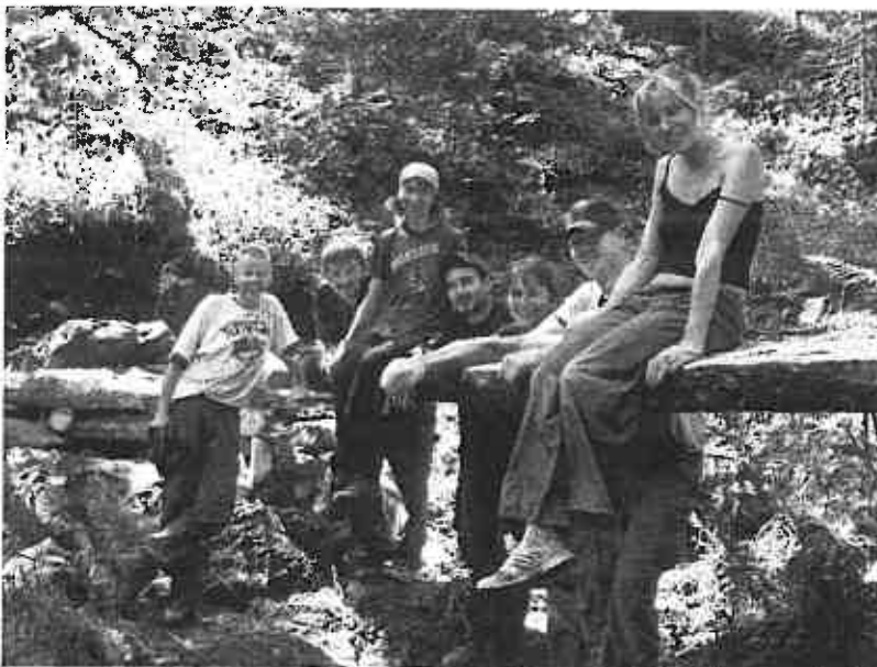
International GBT volunteers take a rest on the bridge we built together. Represented in this photo are Russia, Germany, Canada and the United States.
