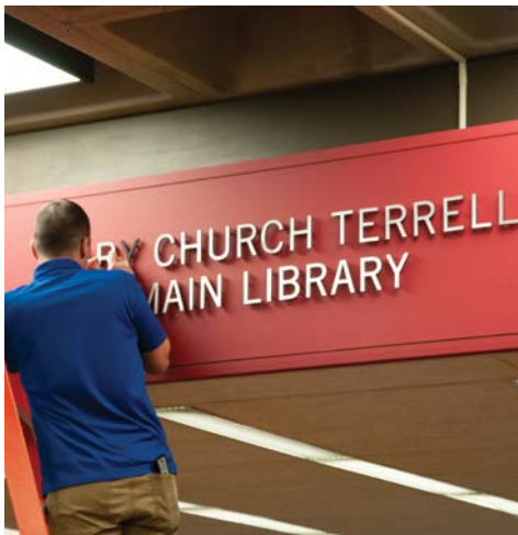
Installing the aluminum letters “Mary Church Terrell Main Library” in the Academic Commons
