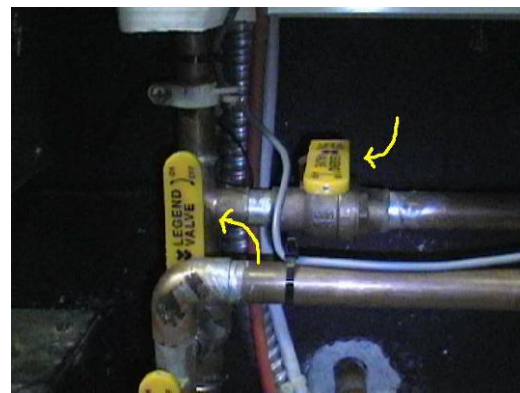
2. Air Gap meter is off and water flows directly to greenhouse hose.
